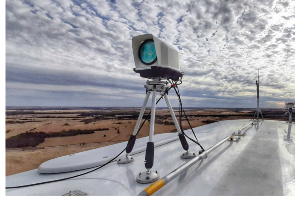
Fig.1 NML installation photo
