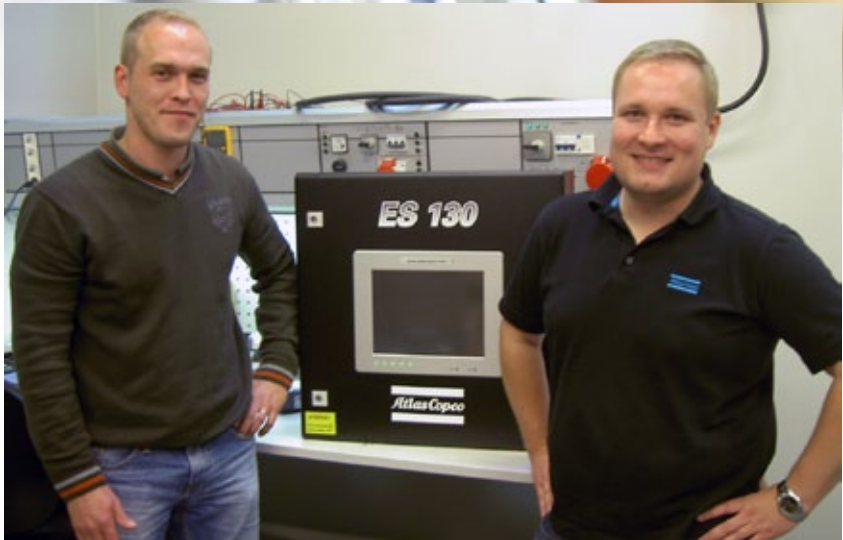
Operational Service Manager Tommy Fagerström and Service Sales Engineer Mika Ikonen present the Atlas Copco ES 130 central controller for compressed air systems. A fixed Vaisala DMT340 is integrated in many of these.
