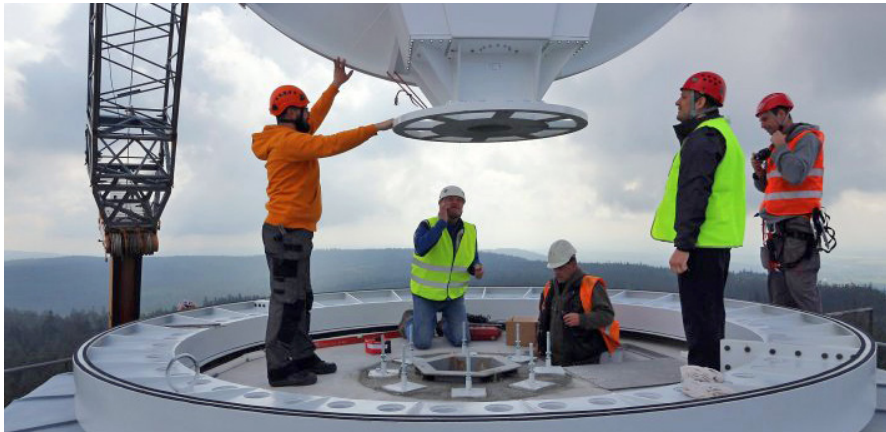
Installation of WRM 200 antenna at Brdy-Praha site
