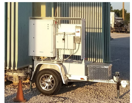
OPT100 Mobile Installed on a transformer.
