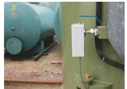
MHT410 prototype installed in radiator pipeline.
