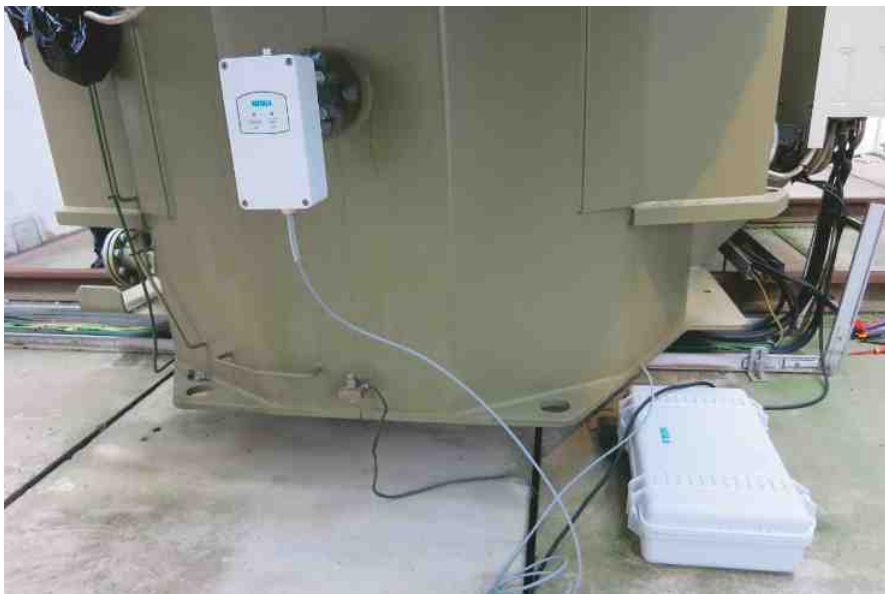
MHT410 prototype installed in instrumentation valve at Vantaan Energia site.
