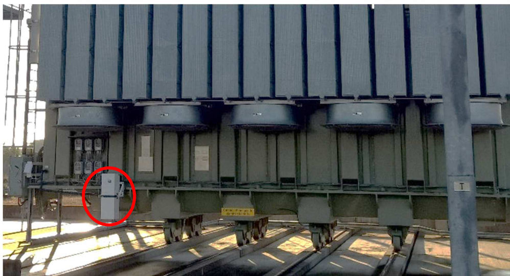
Figure 3 400 MVA transformer with Vaisala online DGA-monitor prototype (red circle).
