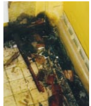
Water had damaged the wall in the washroom.
