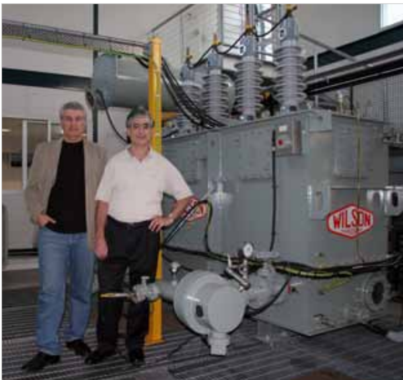
Dr. Valery Davydov and Dr. Oleg Roizman in front of the transformerLIFE Centre's test transformer.
