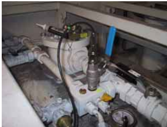
A HMP228 unit installed in a ship's machine room. Installation is easy and convenient to perform through a ball valve.
