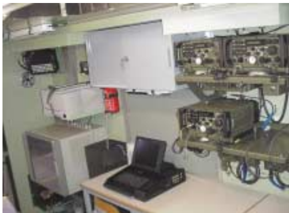
The sounding workstation and telecommunications equipment are operated inside the spacious EMI/EMC protected shelter.
