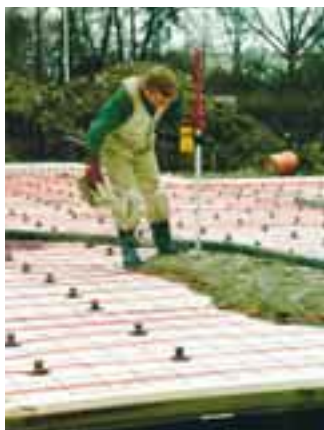
In new construction, the tight time schedule may not allow enough time for structures to dry completely.
