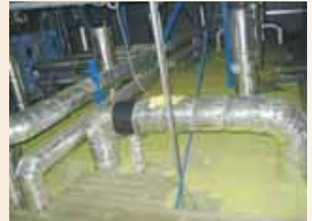
The measurement drum was located in the loft of the wood dryer compartment.
