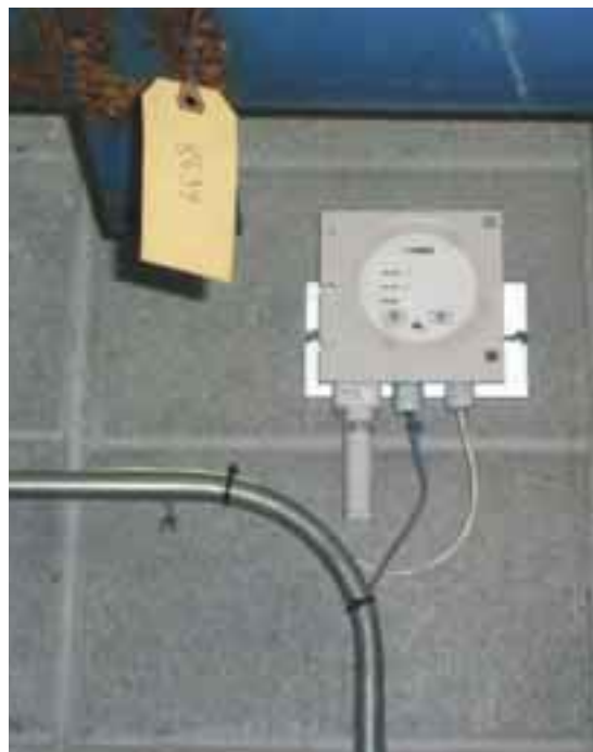
Figure 2. A Vaisala Ammonia Detector AMT102 in operation at the cold storage facility of Associated Wholesale Grocers.
